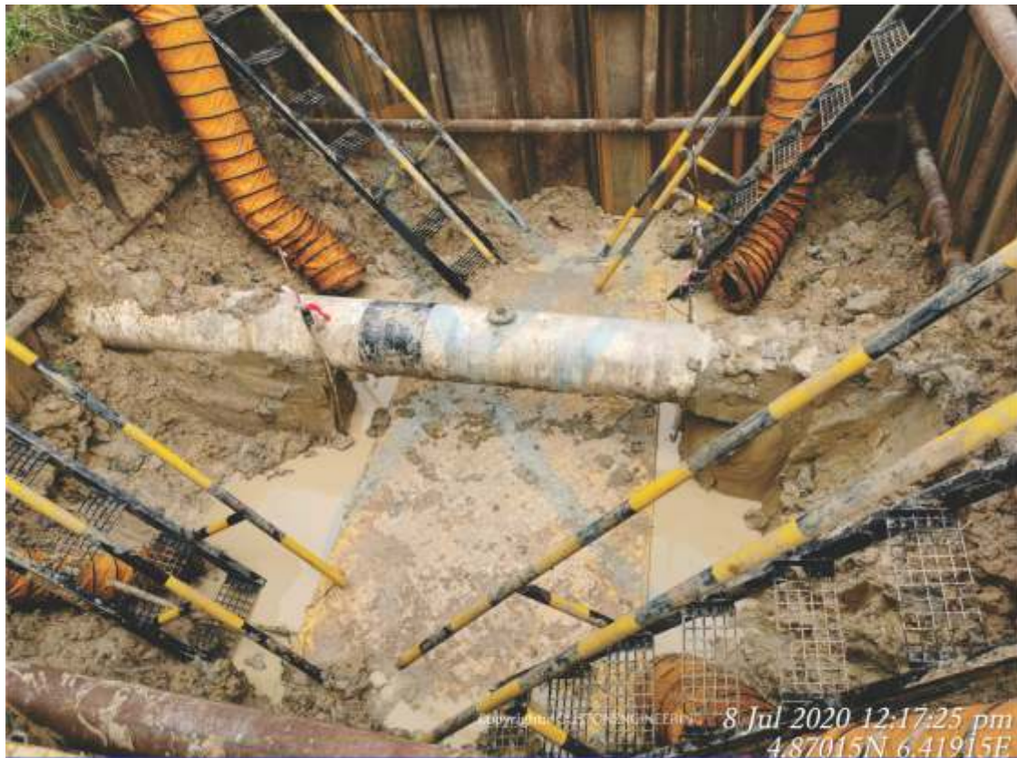
COC ON GAS LEAK REPAIR BY CLAMP WELDING ON 20" KOLO CREEK - SOKU PIPELINE
