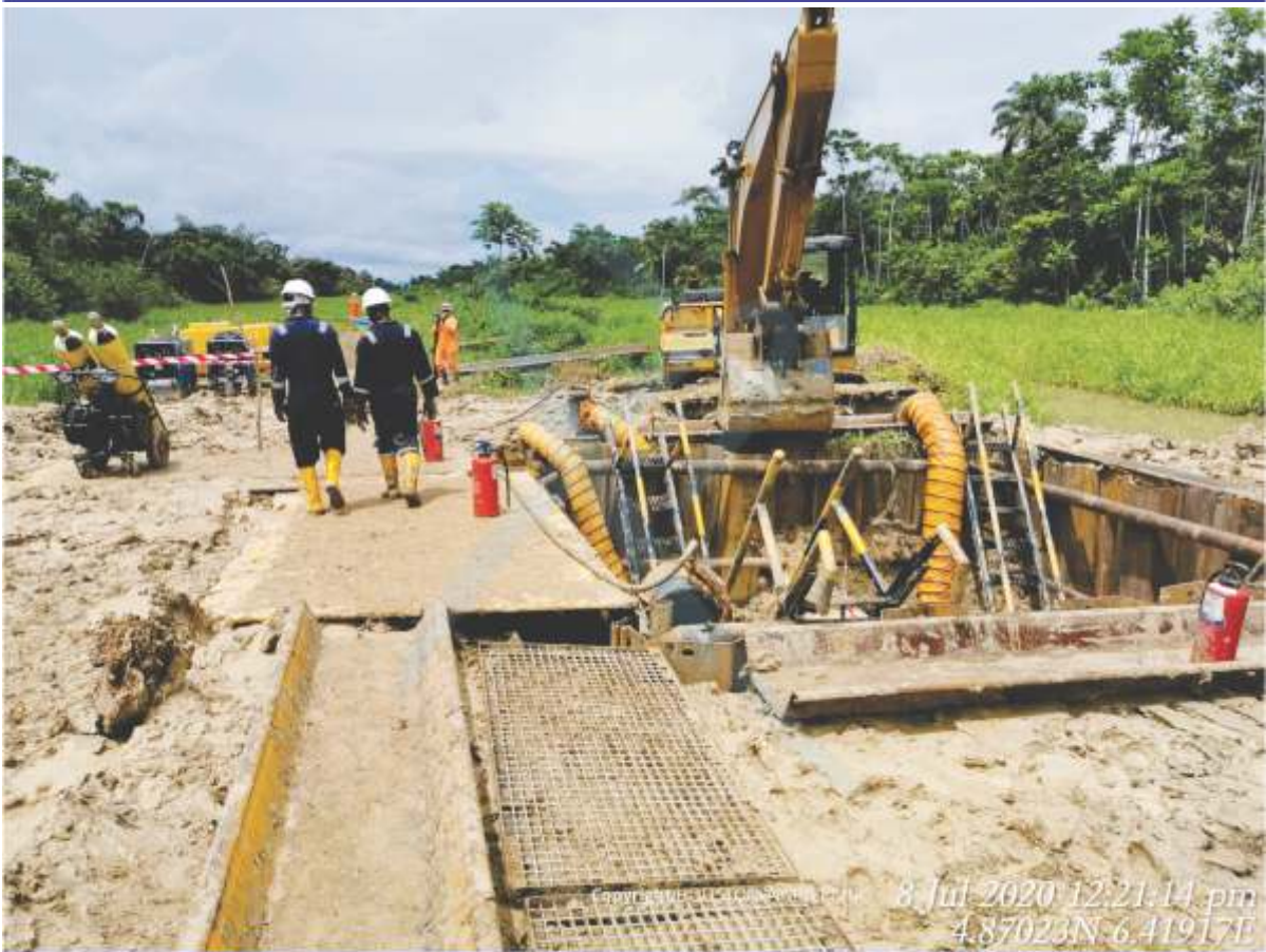
SITE LAYOUT ON GAS LEAK REPAIR BY CLAMP WELDING ON 20" CLAMP ON 20" KOLO CREEK - SOKU PIPELINE
